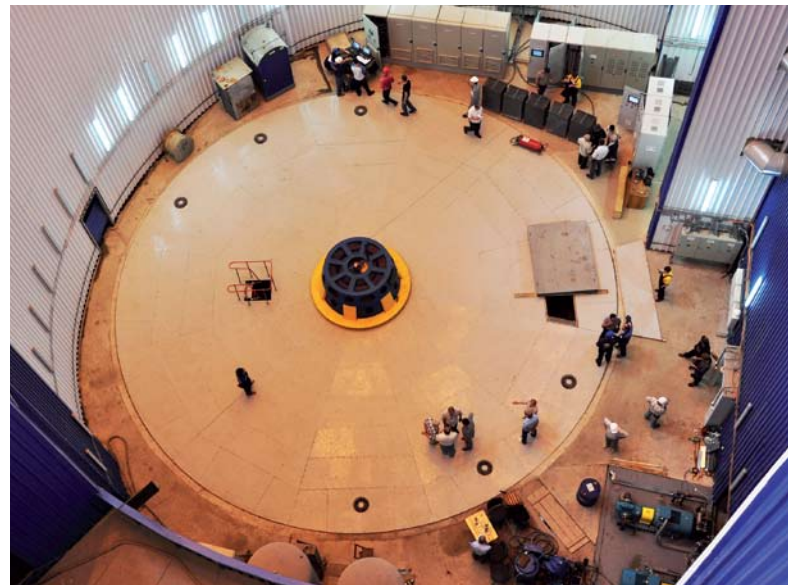
Emerson's Ovation system monitors and controls all major equipment and processes at the Dnestrovskaya pumped storage power plant (PSP)
